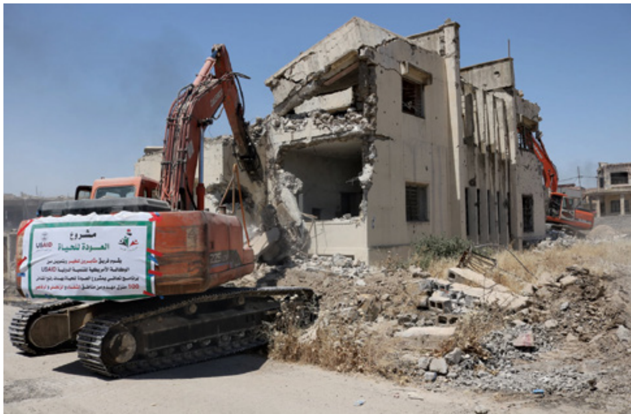
Rubble and debris are removed from demolished homes in neighborhoods in Mosul. (USAID photo)
